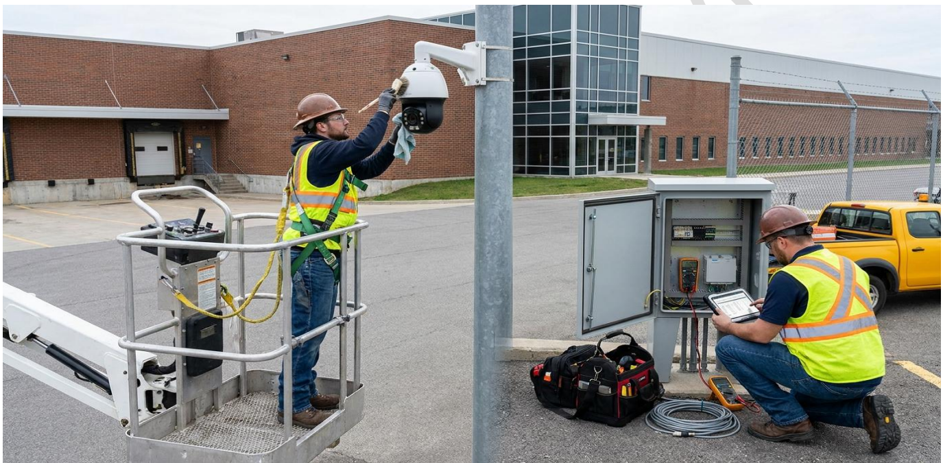
Preventive camera maintenance and field system-health inspection.
