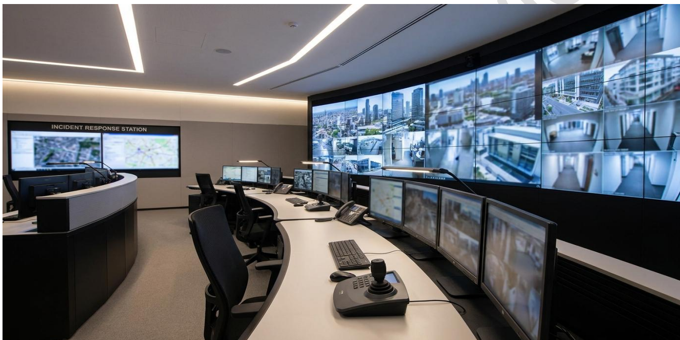
Ergonomic security control room with video wall and PTZ operator controls.
