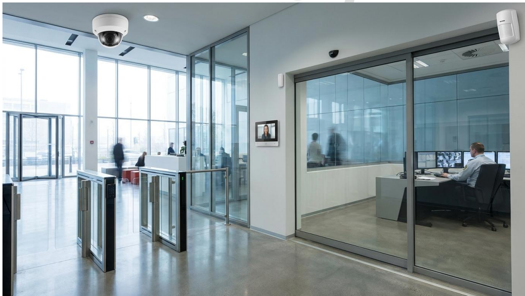
Integrated entrance security with video, access control and intercom.
