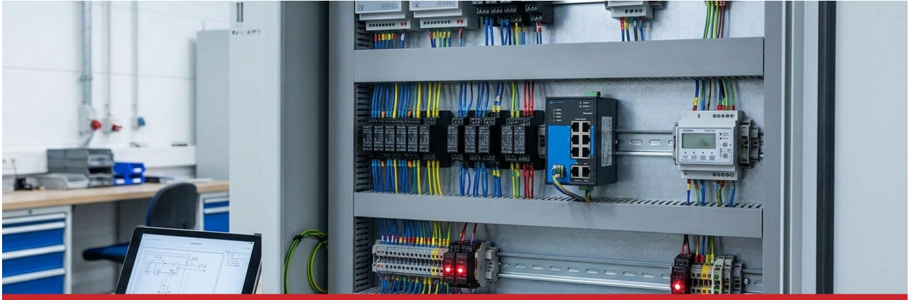
Lighting controllers, gateways, relay modules, network equipment and energy metering
