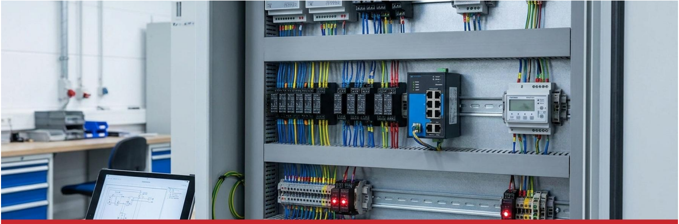
Addressable devices and control points organized for testing, alarms and maintenance
