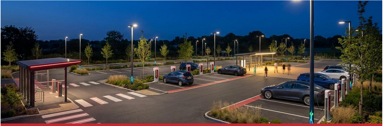
Efficient pole, EV-zone, pedestrian and open-air parking illumination
