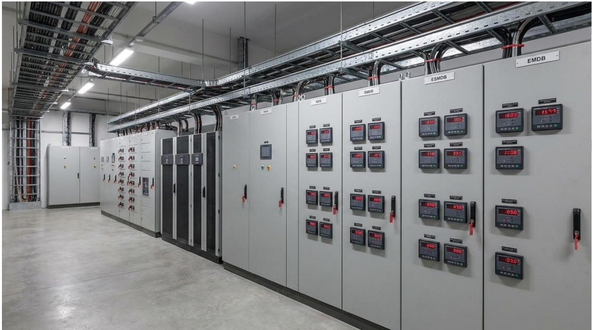
Illustrative integrated electrical equipment room with intelligent metering.
